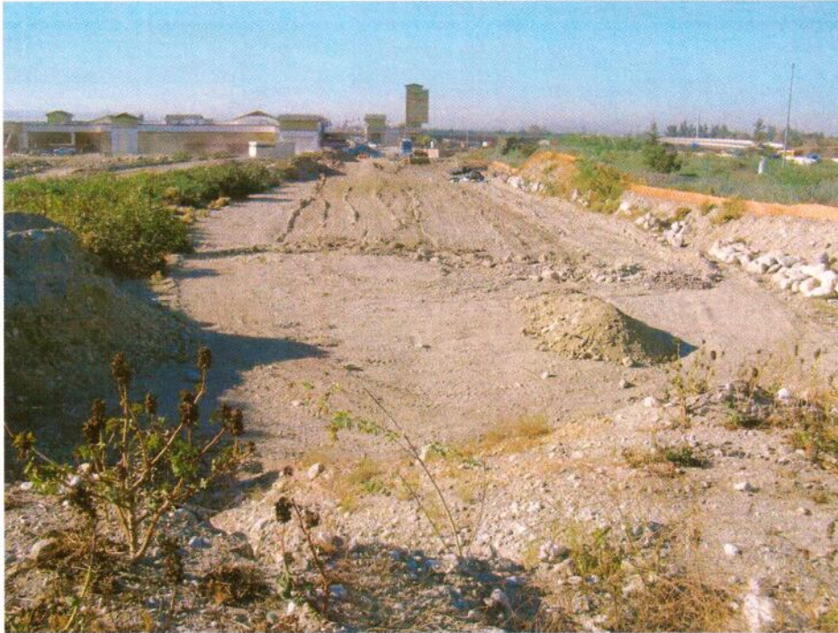
South-facing view of graded area at west end of Planning Area 3 along State Route 210.
